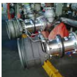
Oil and gas flow control
